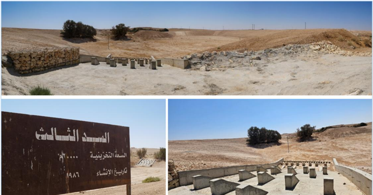
Photos from the field visits showing Check Dams, in Muwaqqar Site, Jordan University. At the Muwaqqar Research Station, managed by the University of Jordan, the project constructed a series of check dams as part of its integrated water harvesting system. These low-cost, nature-based structures were designed to slow surface runoff, reduce soil erosion, and recharge groundwater aquifers. By retaining rainwater, check dams improve infiltration and contribute to local aquifer recharge, and the captured water supports surrounding vegetation and experimental plots used for training and demonstration.
