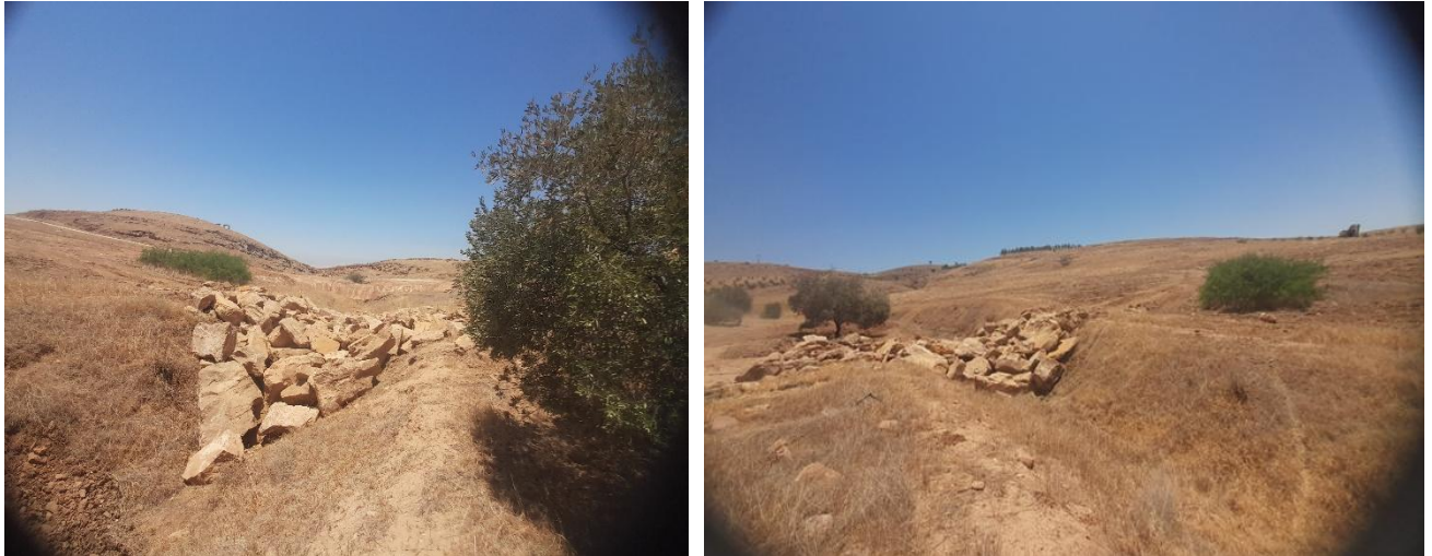
Check Dam and Gully Plug at Humret AL Sahen.
