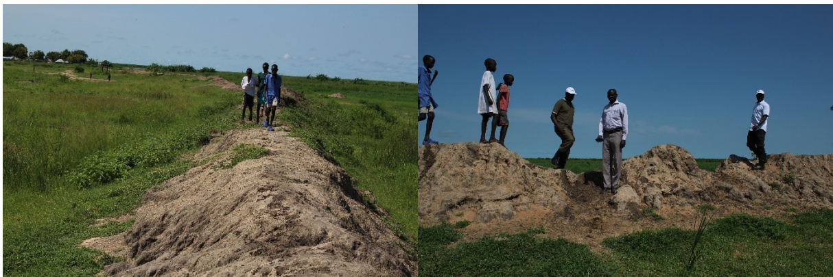
Photo 1: Overall dyke along the Nile in north-west of town, with damage by livestock trampling
