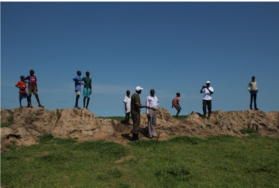
Photo 14: Earthen dyke, northern Bor, damaged by cattle
